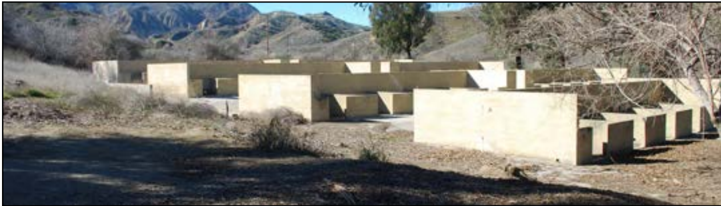
Existing masonry horse corrals should be demolished.
